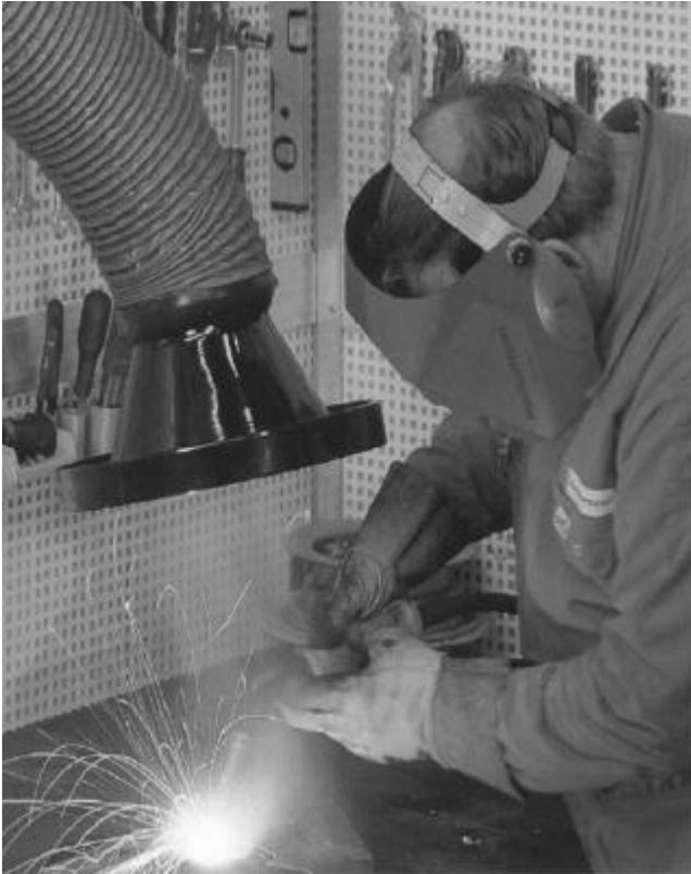
Welding Fumes Extraction
